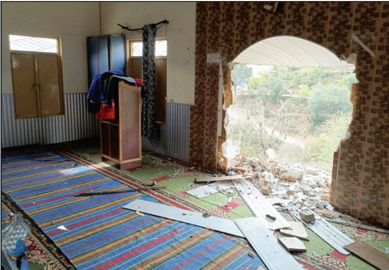
Mosque wall destroyed
