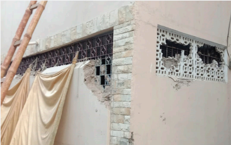
Damage to outer structure
